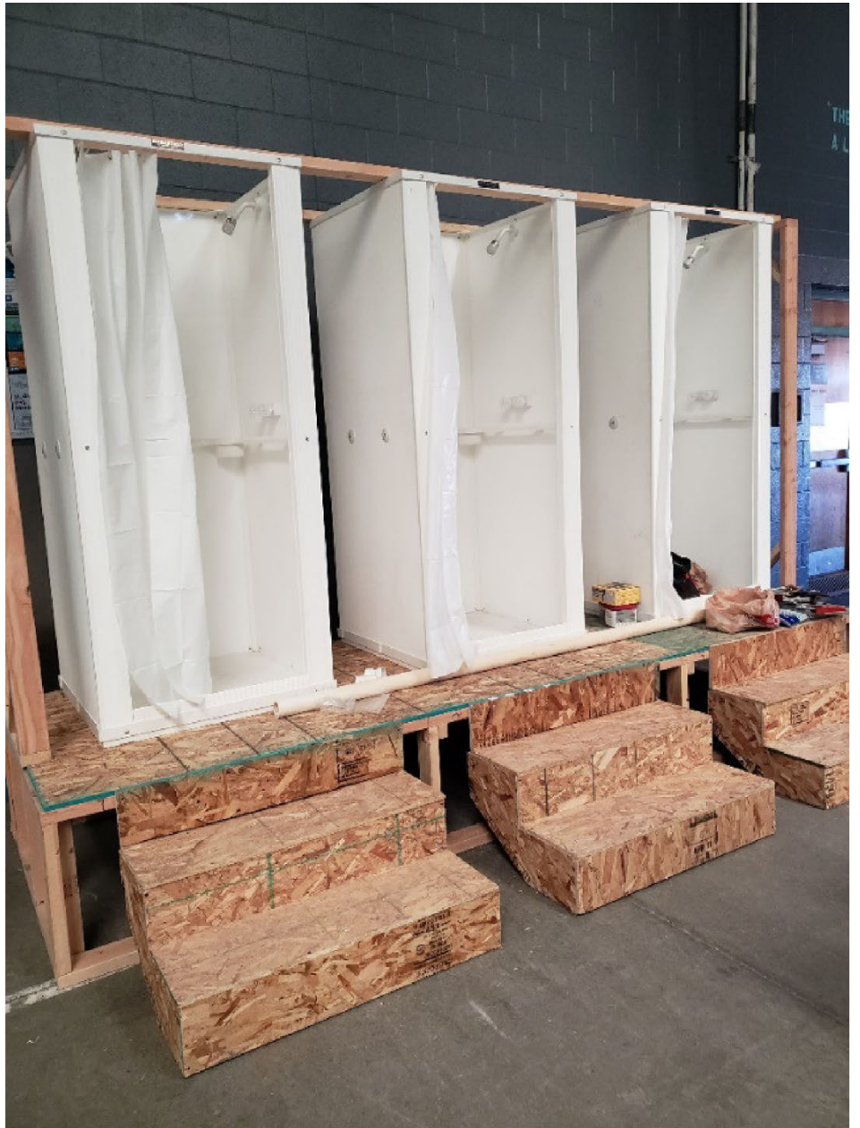
Figure 14: A Federal Bureau of Prisons Facility's Installation of Temporary Showers in Alternate Housing Areas for Inmates in Quarantine and Isolation
