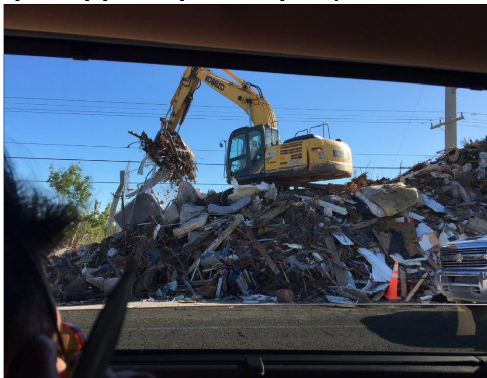
Figure 29: Staging Debris along Route 1 near Big Pine Key, Florida October 2017
