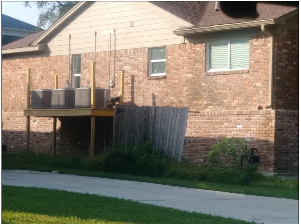
Figure 31: Elevated Air Conditioning Unit in Greater Houston Area, October 2017
