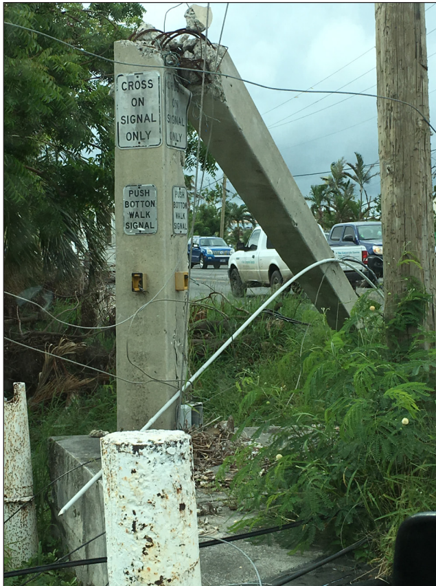
Figure 9: Damaged Power Pole in the U.S. Virgin Islands after Hurricane Maria in November 2017
