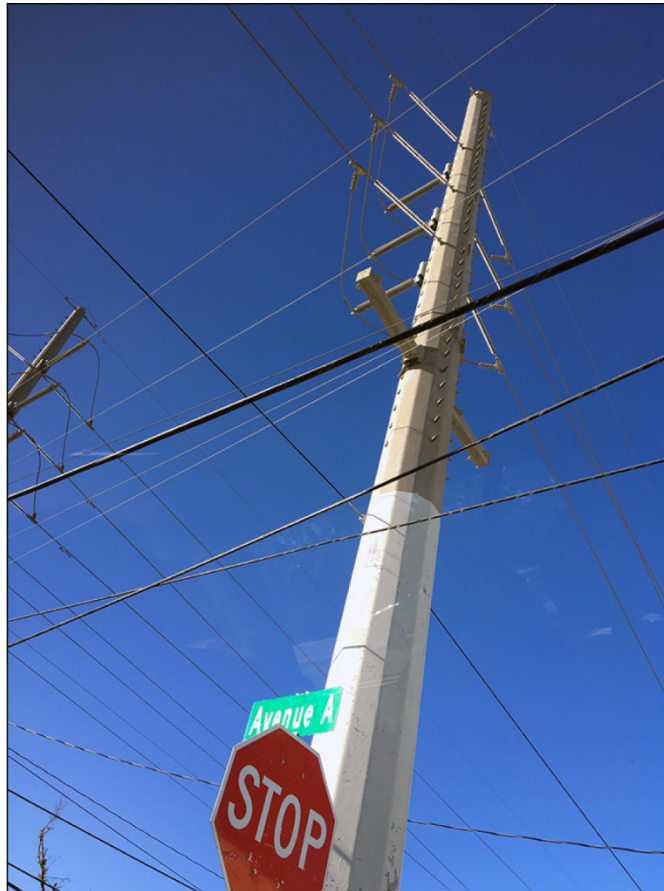
Figure 32: Reinforced Power Line Poles in Monroe County, Florida, October 2017— Post Hurricane Irma
