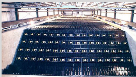
Sources: GAO analysis of DOE documents and data and interviews with DOE officials. Image source: DOE. | GAO-17-306
