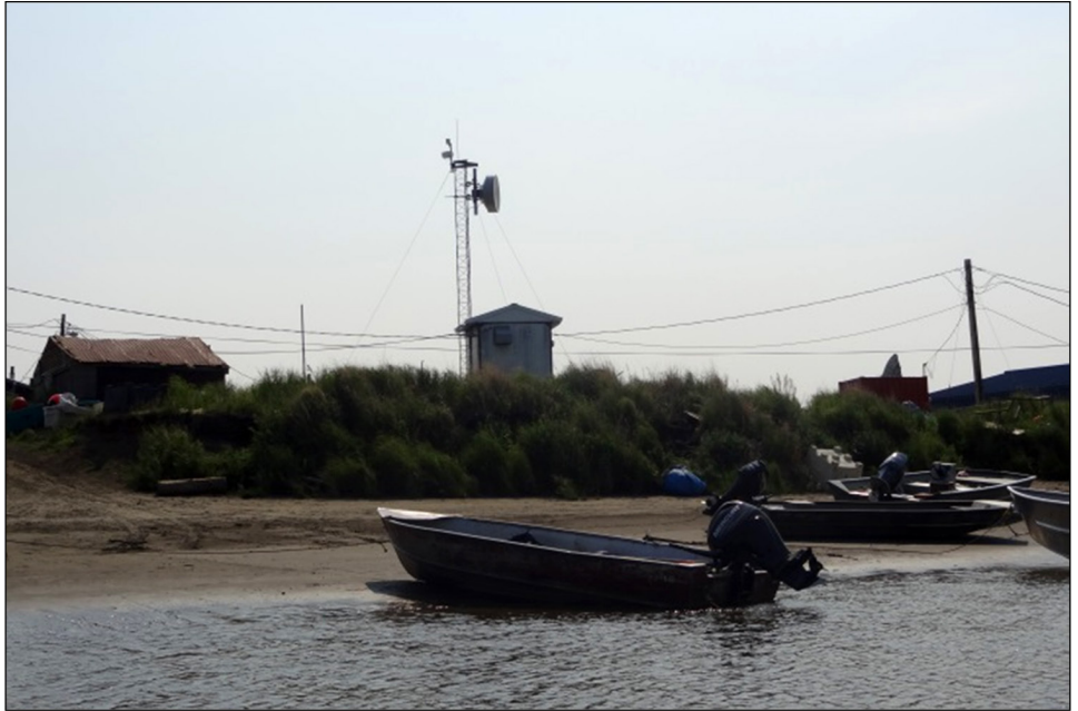
Figure 6: Wireless Microwave Internet Tower in Oscarville, Alaska
