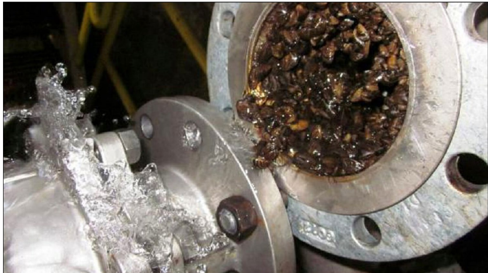
Figure 2: Zebra Mussels Clogging a Pipe
