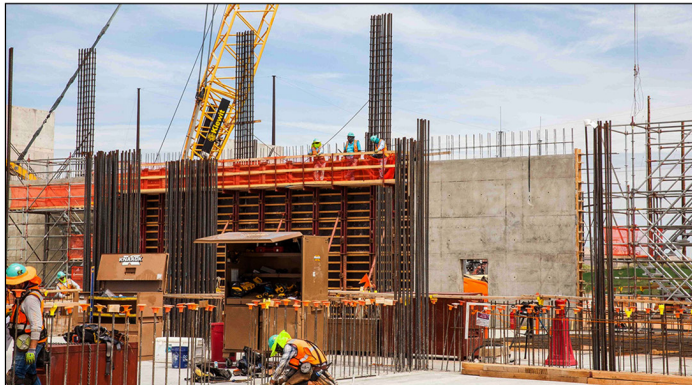
The Department of Energy's (DOE) Ventilation System Project at the Waste Isolation Pilot Plant in New Mexico
