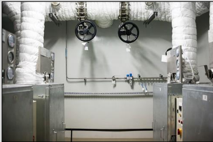
Example of insulation at an industrial facility
