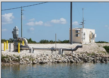
Well used to adjust salinity in the Turkey Point Nuclear Generating Station's cooling canals
