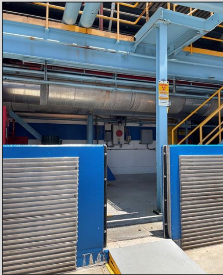
Flood barrier protecting part of the Turkey Point Nuclear Generating Station
