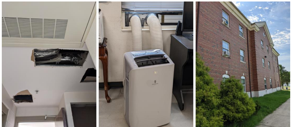
Figure 4: Broken and Supplemental Air Conditioning Systems
