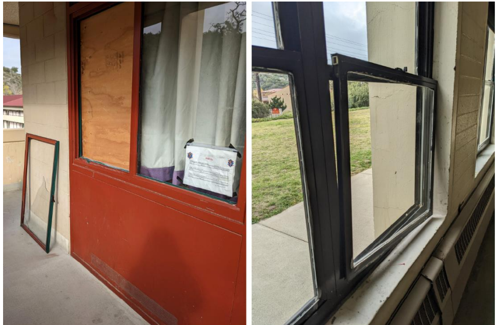
Figure 10: Broken Windows Observed during GAO Site Visits
