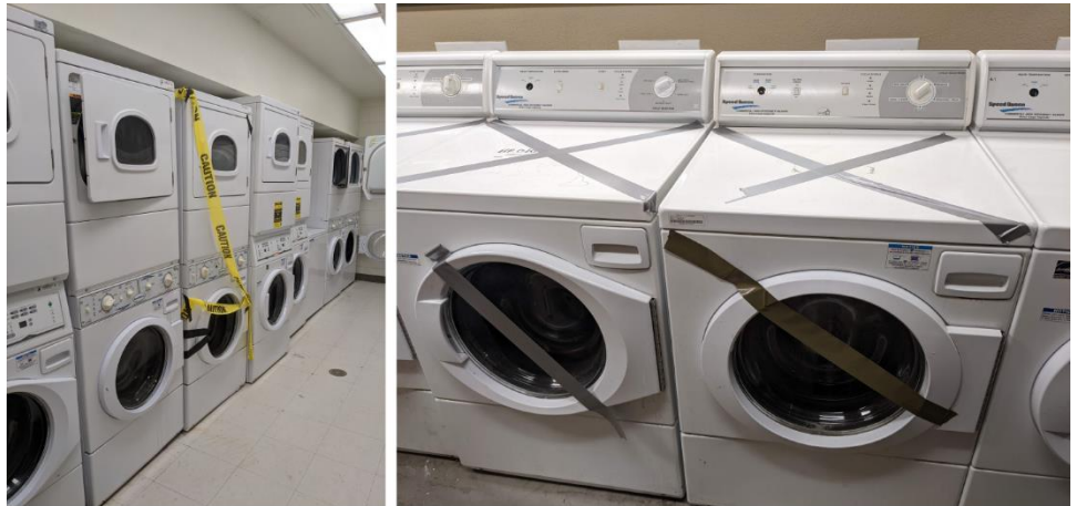
Figure 21: Broken Washing Machines and Dryers at Military Installations
