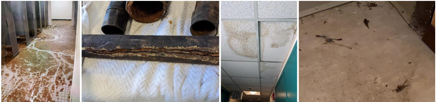
Sewage overflow in training barracks restroom
