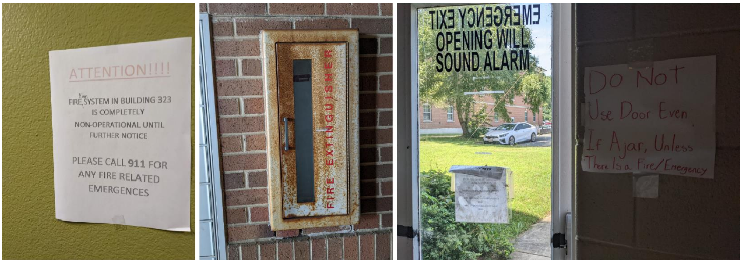
Figure 9: Fire Safety Issues Observed during GAO Site Visits
