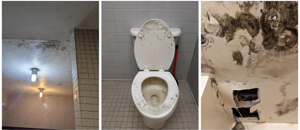
Figure 7: Mold in Barracks Observed during GAO Site Visits
