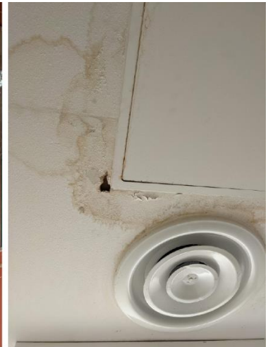
Ceiling water damage due to broken heating, ventilation, and air conditioning system
