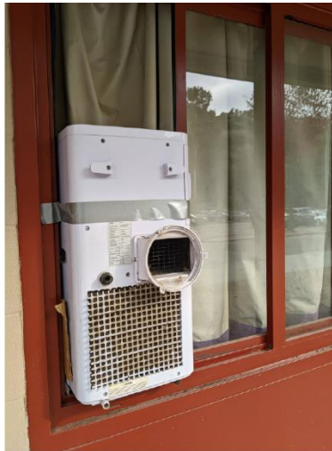
Window air conditioning unit installed in barracks with broken central air conditioning
