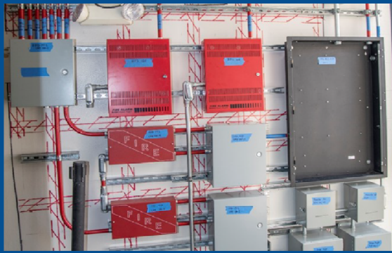
Source: Work performed for Department of Energy. | GAO-23-104402
