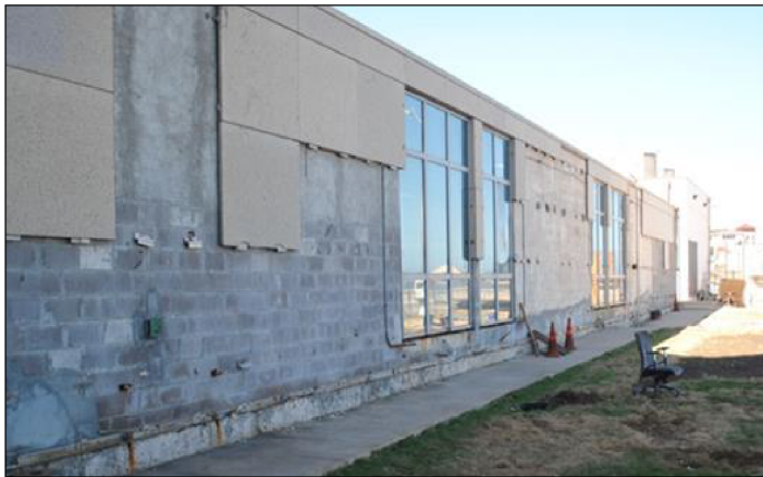
Damage to exterior walls.
