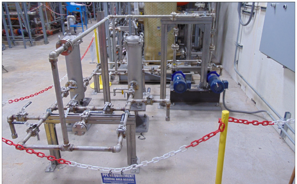
Figure 5: Example of Pipe Upgrade at the Paducah DUF6 Conversion Facility Pipes carrying potassium hydroxide—used to neutralize hydrofluoric acid during the depleted uranium hexafluoride (DUF6) conversion process—were originally made from PVC. Officials from the Department of Energy’s (DOE) Office of Environmental Management (EM) replaced the PVC pipes with stainless steel.
