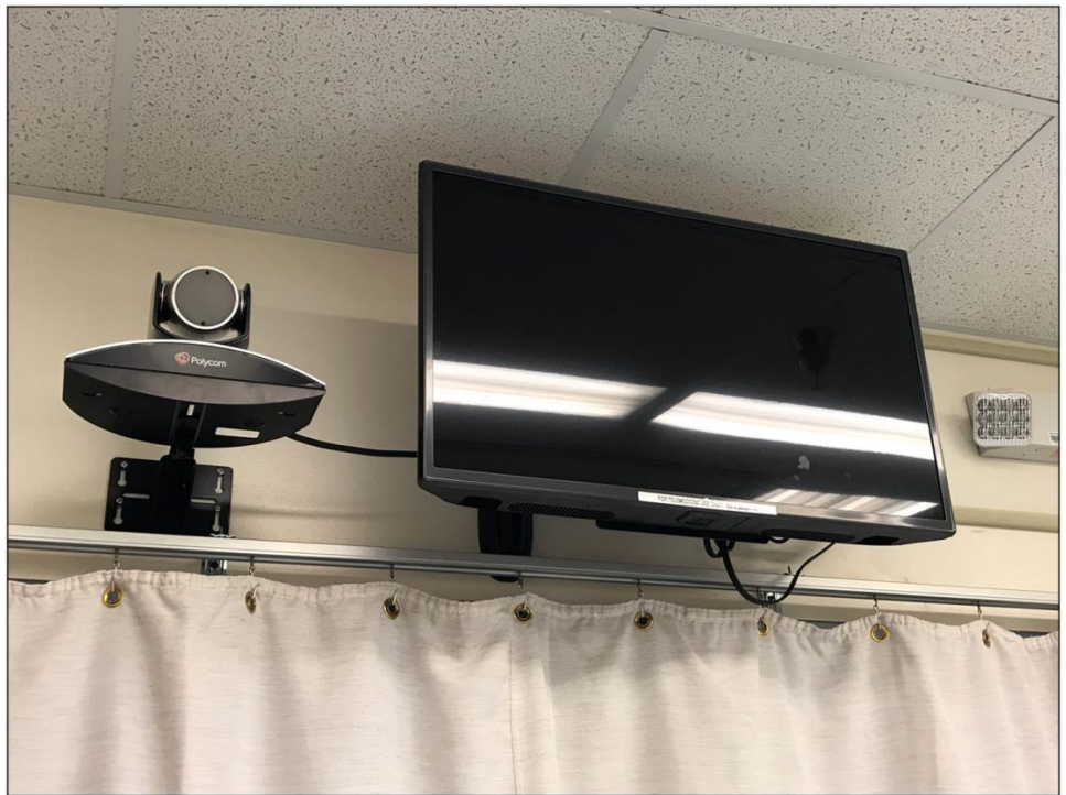
Figure 7: Telehealth Equipment in the Rosebud Hospital Emergency Department
